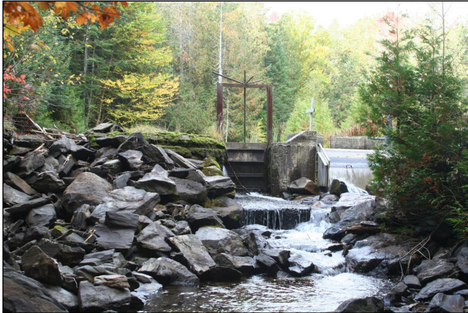
Figure 32. The upper Bald Hill Fish Hatchery dam (State ID 137.07) poses a formidable barrier to aquatic organism passage in Bean Brook.
